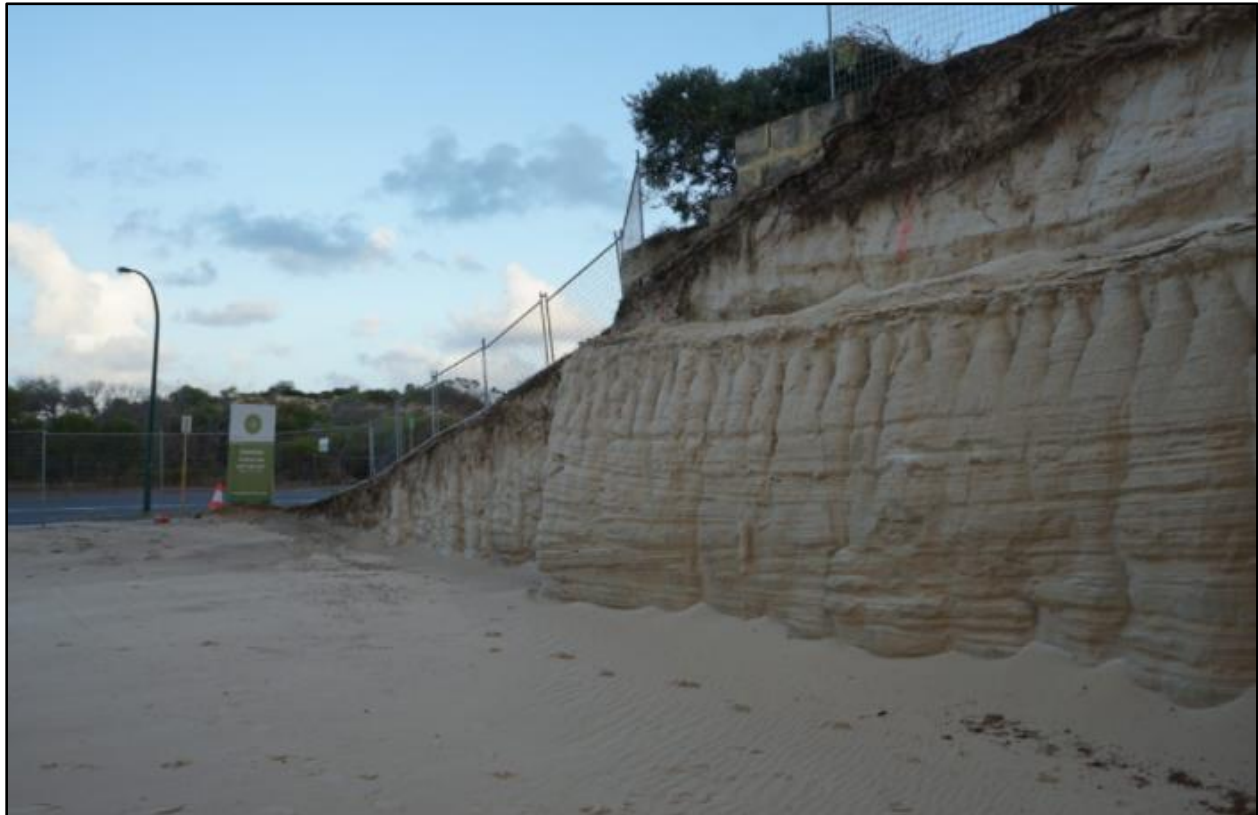
Figure 3-9. Exposed Permeation Grouting in Sandy Soils
